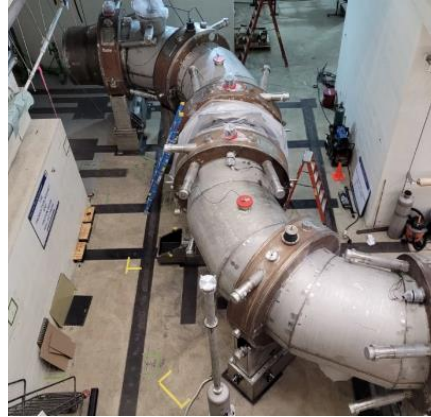
Transport Solenoid: Installed in Mu2e Hall in 2024
