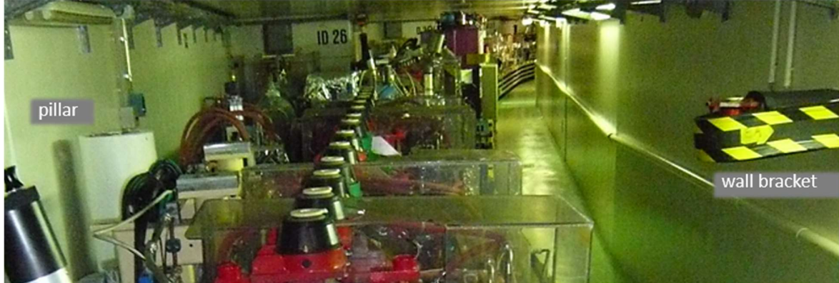
Figure 3 View of the old SR tunnel showing the pillar wall bracket secondary network and the machine. Just to the left of the inscription ID26 is a (closed) window penetration between the SR and the ID26 beamline.
