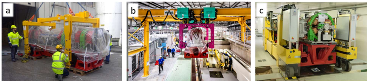
Figure 8 On the left (a), the assembled girder being offloaded from the lorry before final installation. In the middle (b), the girder being lifted over the tunnel wall. On the right (c), the girder being transported to its installation point using the specialised transportation unit.
