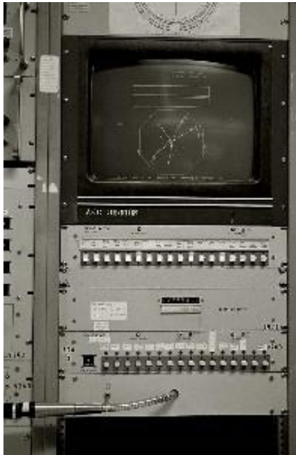
The epicenter of the Control Room.
