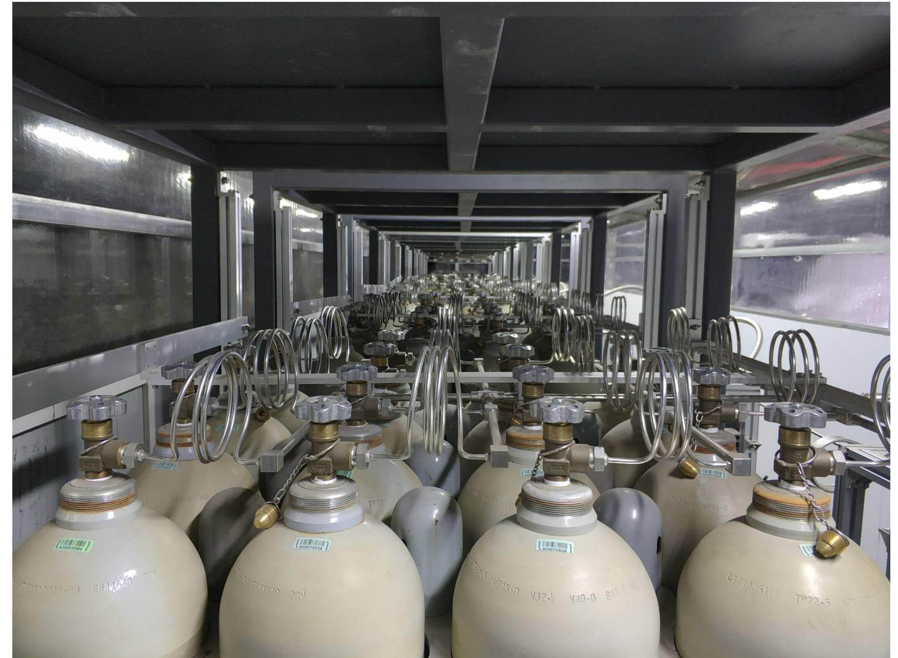
8 modules \times 16 cylinders, 50 kg / cylinder
