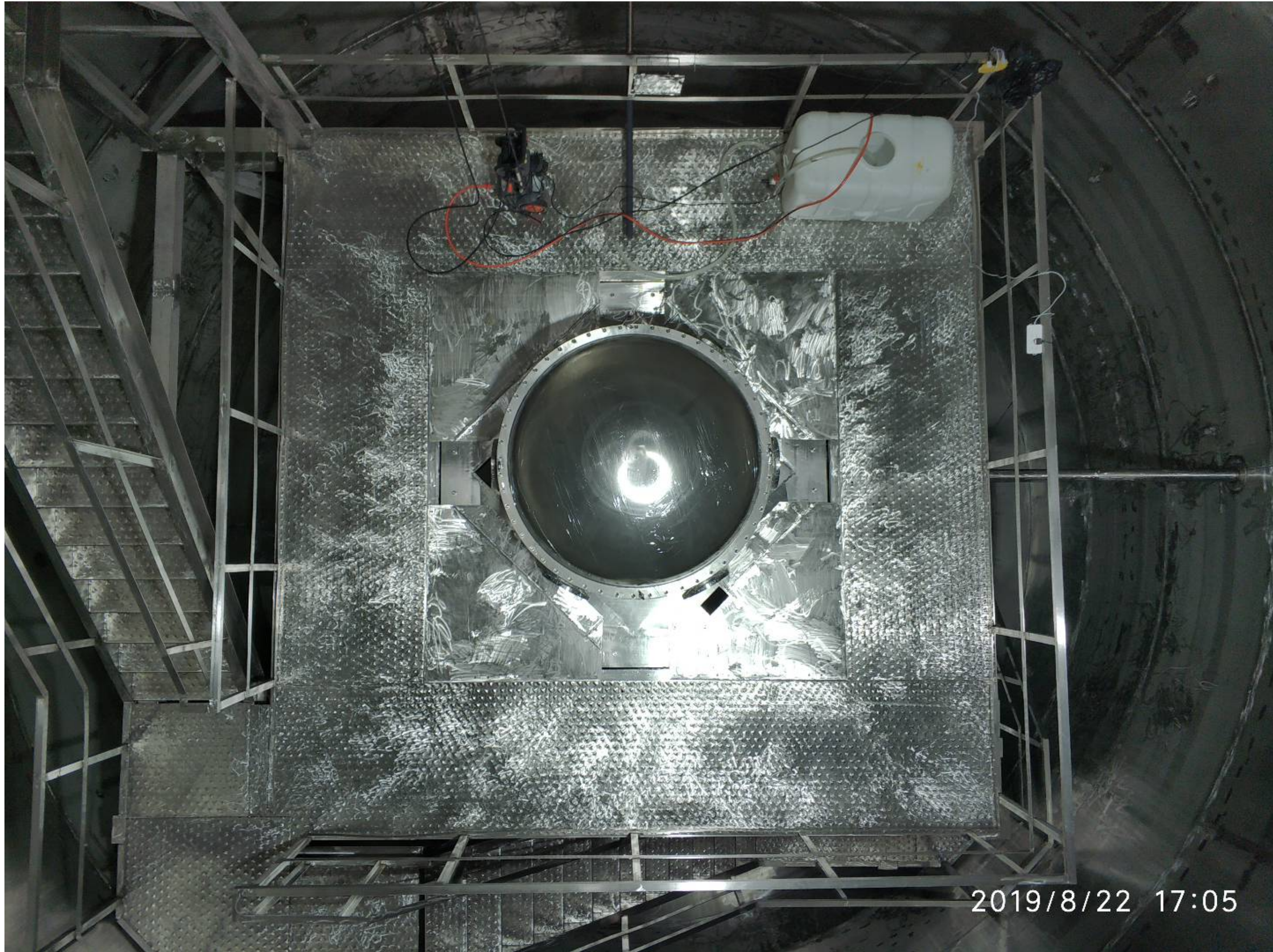
bare stainless steel platform
