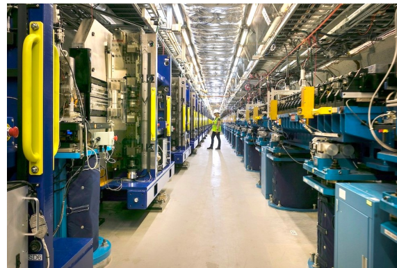
LCLS-II Undulator Hall
