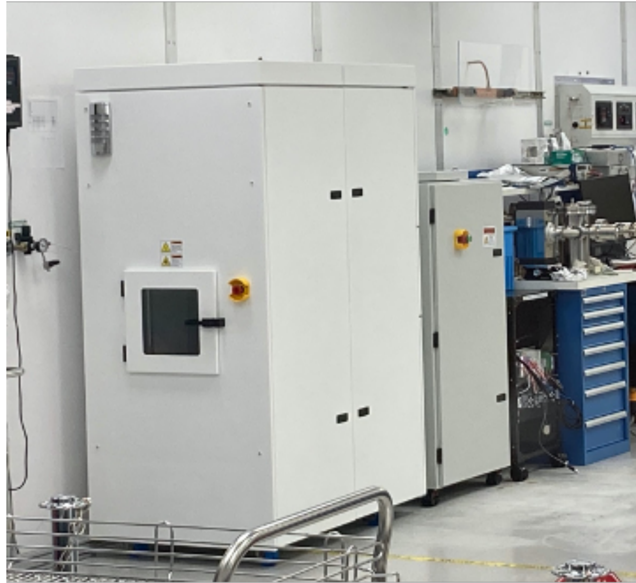
AXOM Microwave Annealing System in SLAC cleanroom
