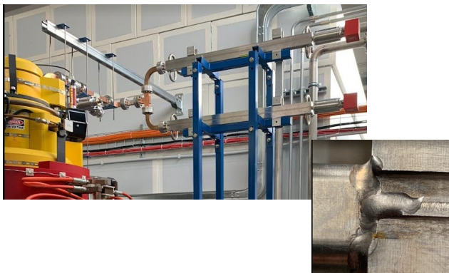
A) RF load: leak check.
