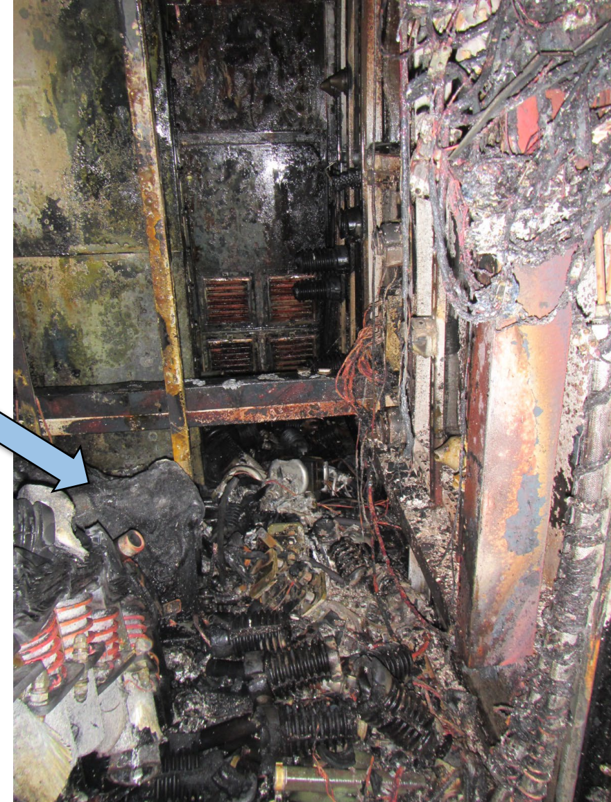
All the plastic-case capacitors meltdown
