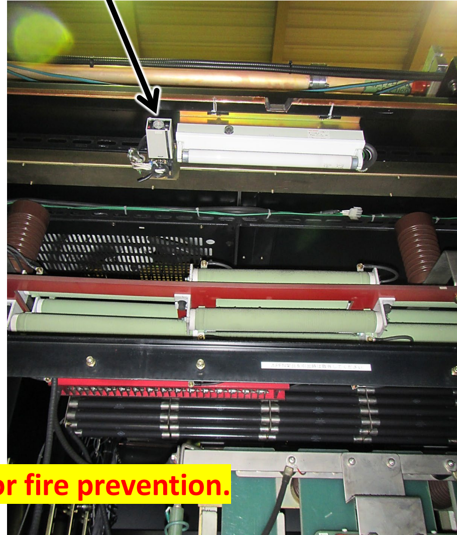
Temperature sensor (Threshold: 40 degC) located at the edge of the ceiling
