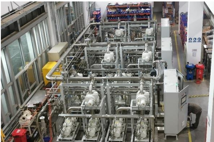
Cryogenic system hall
