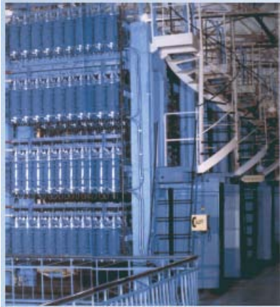
Enrichment to >86% at Electro-Chemical Plant (ECP) in Russia
