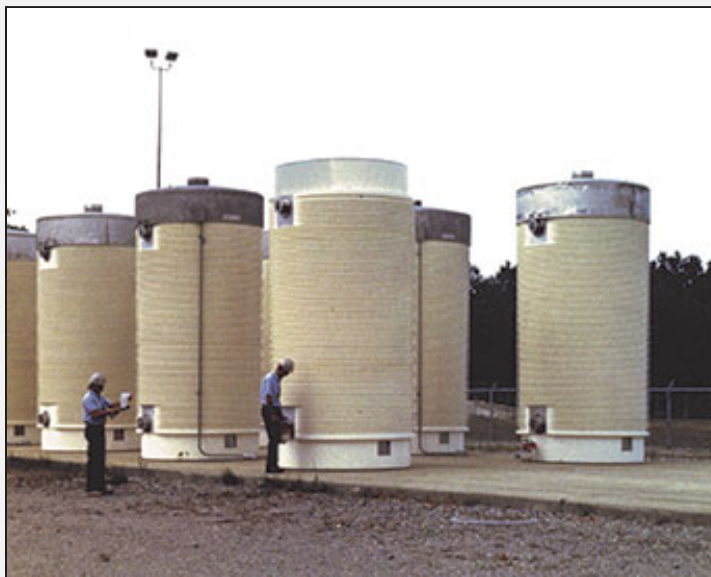
Dry storage casks — sealed, passive, and effectively opaque to conventional re-verification.
